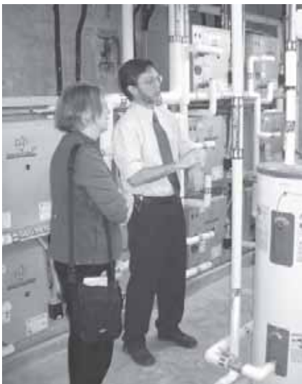
Ned Stowe shows Ruah the controls that provide heating and cooling with water circulated through a deep well.
