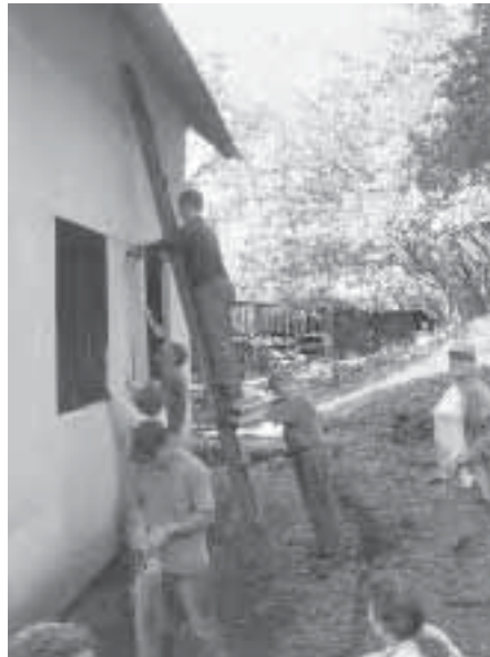
Barbara Williamson, right, supervises work on La Casa Maple , the farm's new community building.
